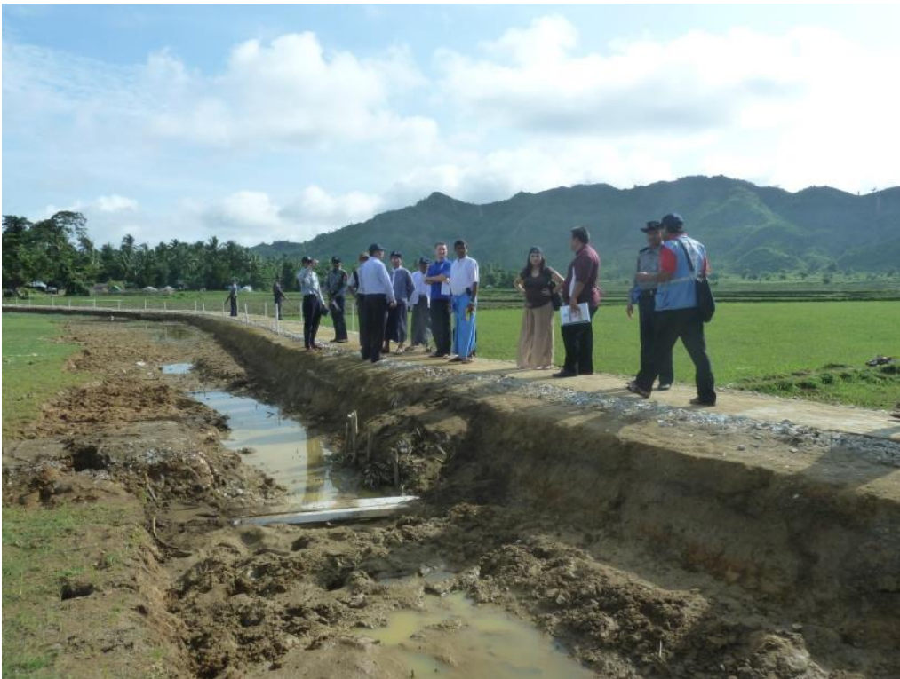
Embankment Construction in Sin Tat Maw Village of Pauktaw Township (Rakhine State)
